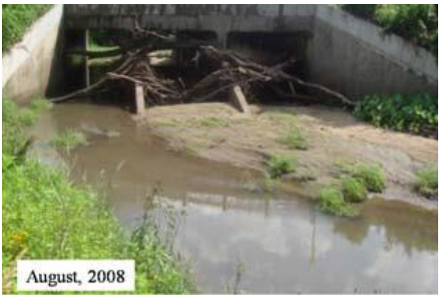
Figure C.1 Sediment and vegetation partially blocking a three-box culvert (Muste, 2009)
